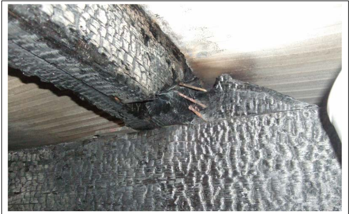
Figure 6 – charring of roof support portal at position of maximum fire intensity
