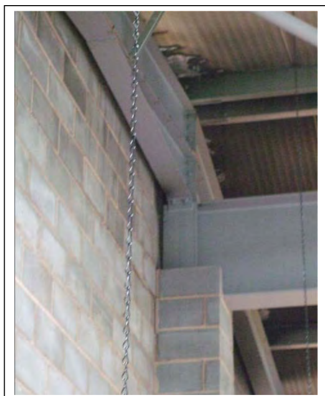
Figure 8 - photograph of underside of roof in Joinery Company demise
