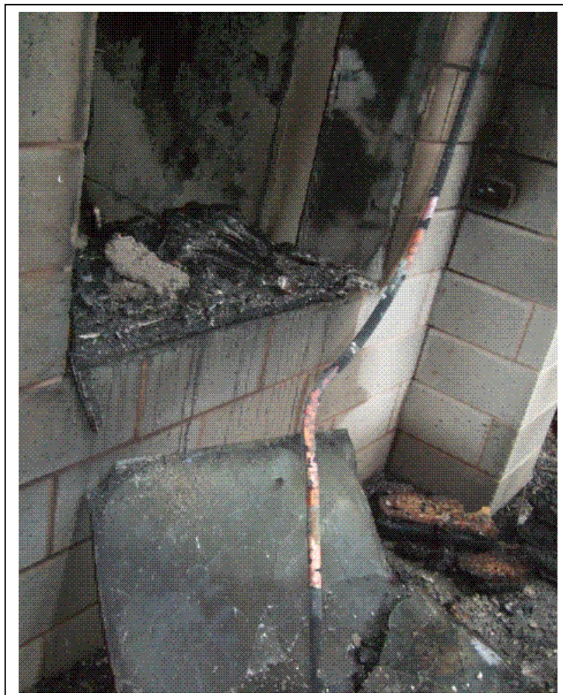
Figure 6 - Effects on fire resisting glazed screen between office and production area
